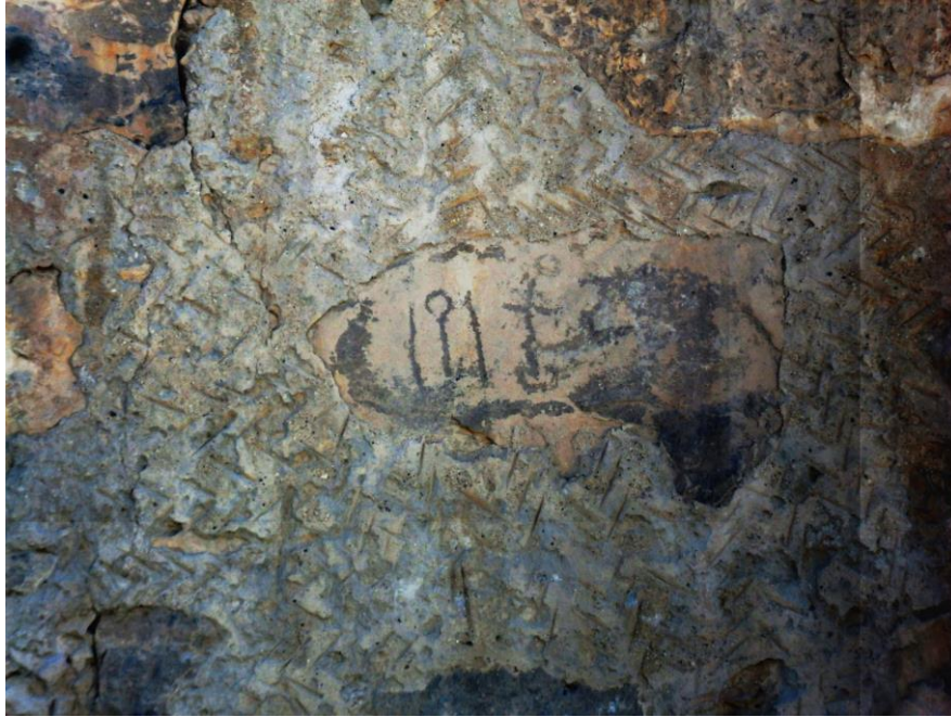
Fig. 2. The marks on the upstream dam (Campana, 2011).
